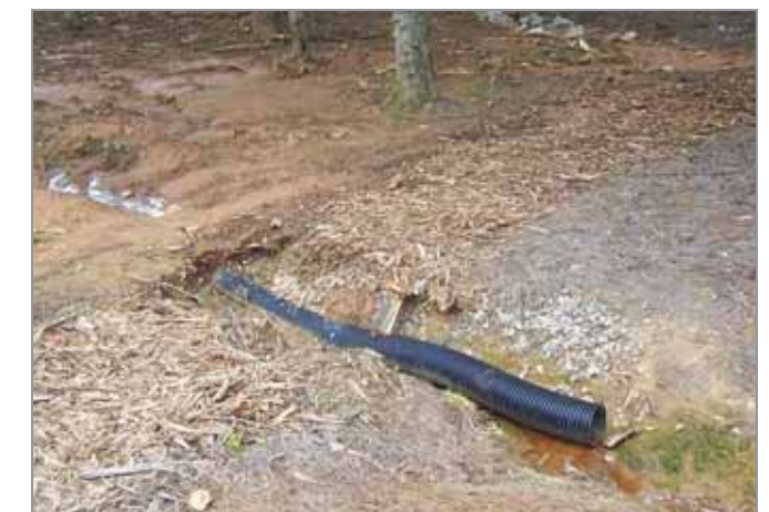
✗ Wood chips can become displaced after rain events, and should not be used for stormwater drainage.
