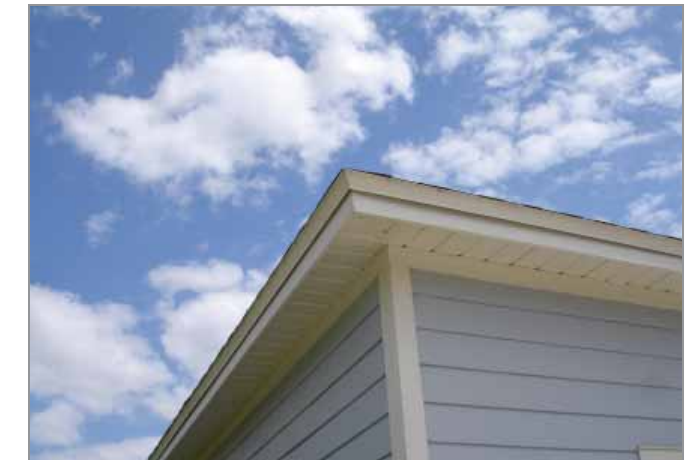
✓ Exposed rafter ends (or tabs) at overhangs are discouraged.
