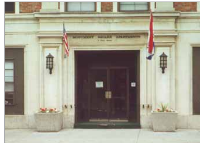
✗ One step at this public building prevents visitors with disabilities to enter
