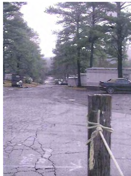
10 - Poor Infrastructure Within Park
